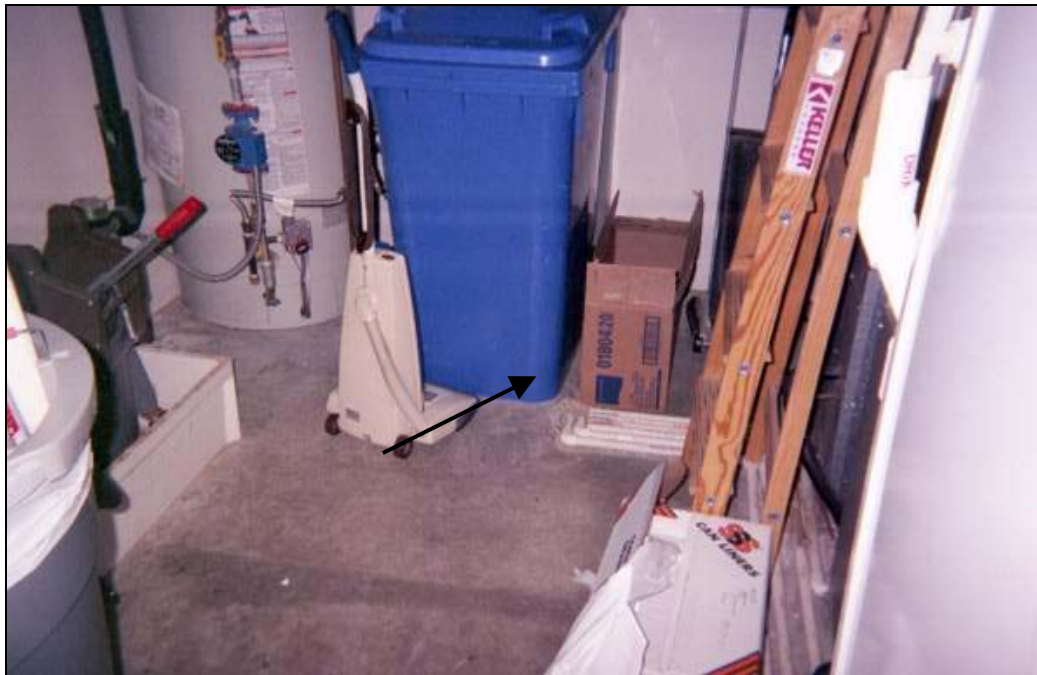
Photograph 2 Furnace Room where Drain Clogged and Water Collected on Floor
